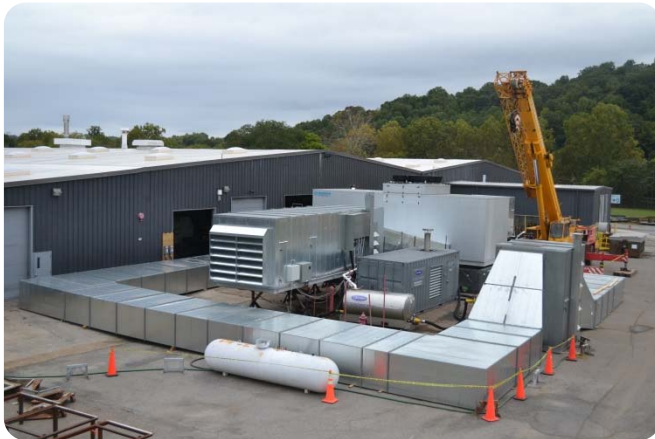
External Test Facility - Virginia
