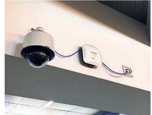
Photo taken at McCarran Airport in Las Vegas – Anyone could jump up and pull out the patch cord to the surveillance camera and wireless access point.
