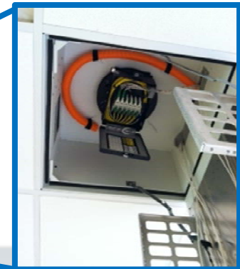
Consolidation Point Zone Cabling
