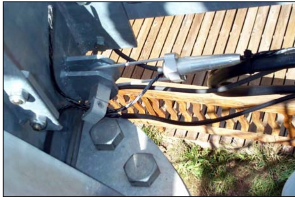
Grounding for communications cable
