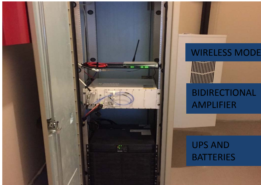
ALL EQUIPMENT IN A SINGLE RACK
