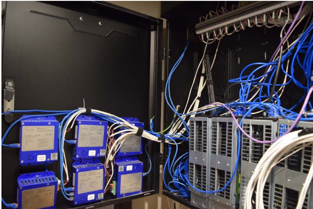
Typical Hallway Cabinet
