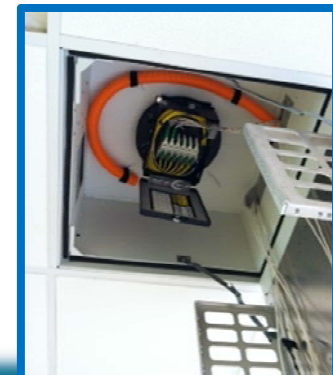
Consolidation Point Zone Cabling
