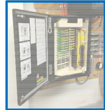
FDH Houses Splitters
