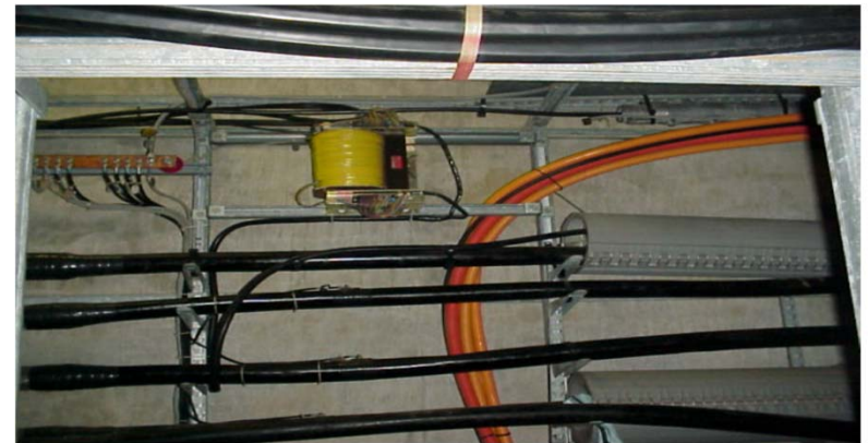
25 Pair INT in Houston AT&T C.O. Cable Vault
