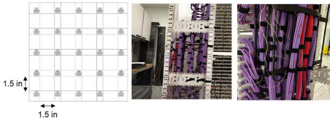
Figure 1 - Example of 28 AWG cord cable bundles consisting of 12 cables separated by a minimum of 1.5 inches in an equipment rack using a 10 inch vertical manager
